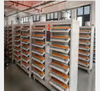
电芯分容 Capacity Grading and Sorting
