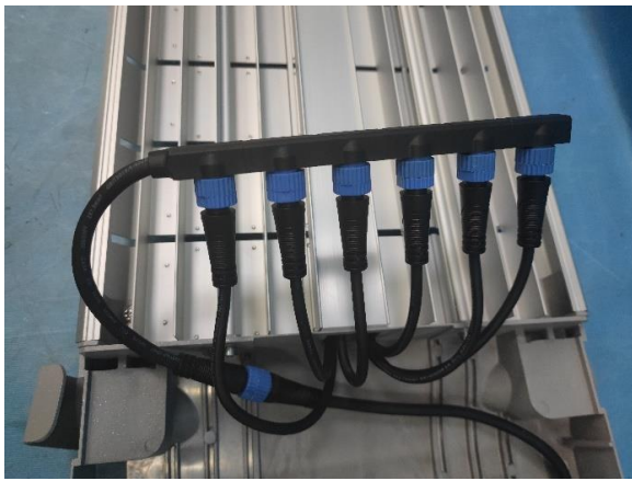
Internal connector wiring
